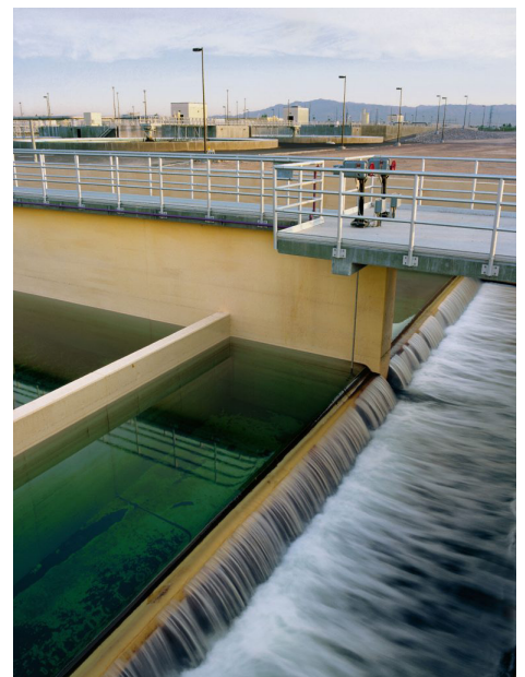
In water treatment applications, turndown is important because the volume and quality of the incoming water can vary on a regular basis.
