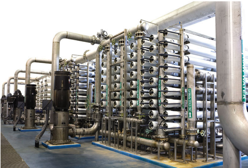
RO skid with membranes. All graphics courtesy of Milton Roy
