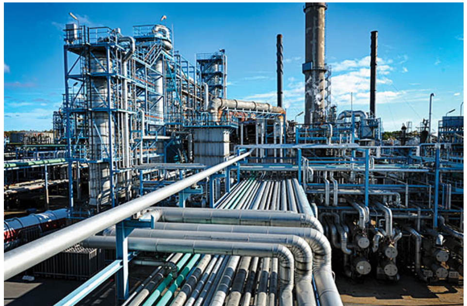
To protect piping infrastructure, scale inhibitors are dosed using metering pumps. Photo courtesy of Pulsafeeder.
