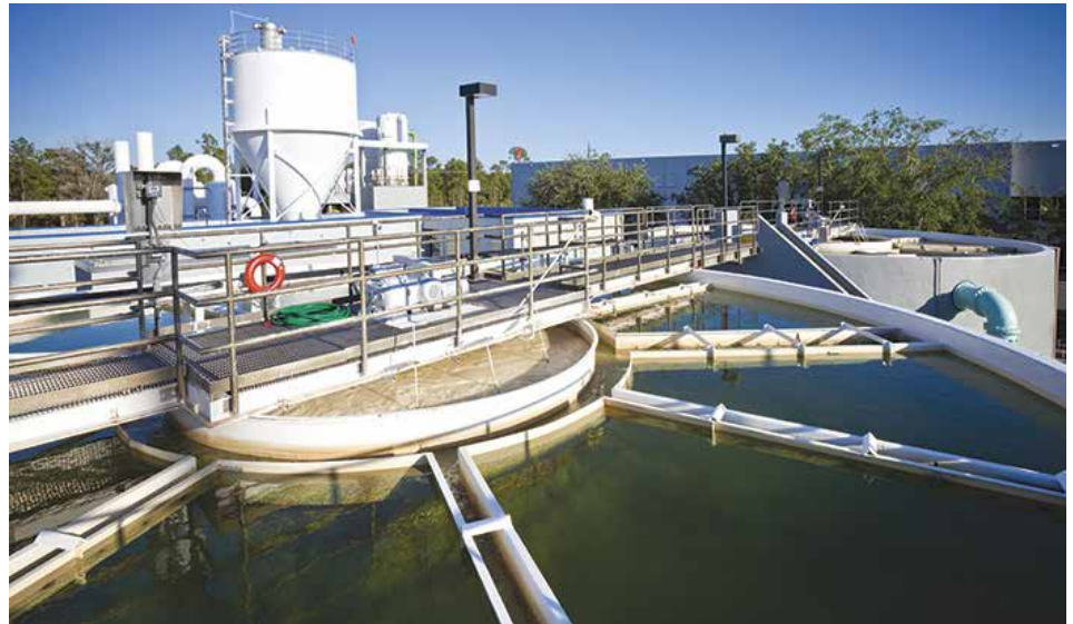
Image 2. Municipal water treatment plants use a combination of reciprocating and rotary pumps for the multiple processes required to make water safe for human consumption.
