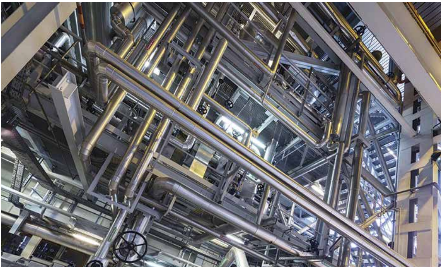
Image 1. It is estimated that almost one-third of all wastewater used in oil and gas production is recycled in some fashion. (Images courtesy of IDEX Corporation)
