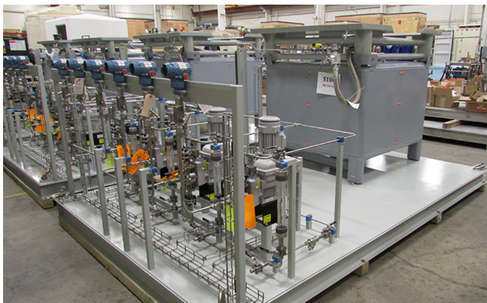
Image 1. AmeriChem Systems Inc.'s chemical feed systems include the pumps, piping infrastructure, valves, flow meters and control systems. (Images courtesy of Pulsafeeder)
